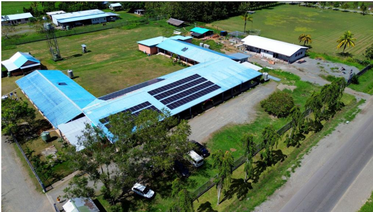
Photo 4 - The hybrid solar-battery-diesel system has produced reliable and free power for the hospital since being switched on.
