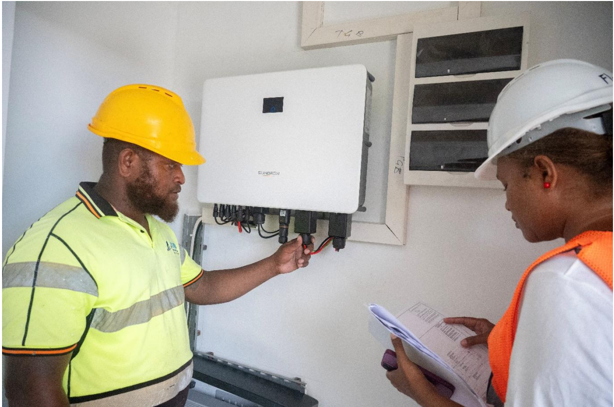
Photo 3 – Australia is working with local suppliers to ensure Solomon Islands has the workforce to install and maintain solar power systems.
