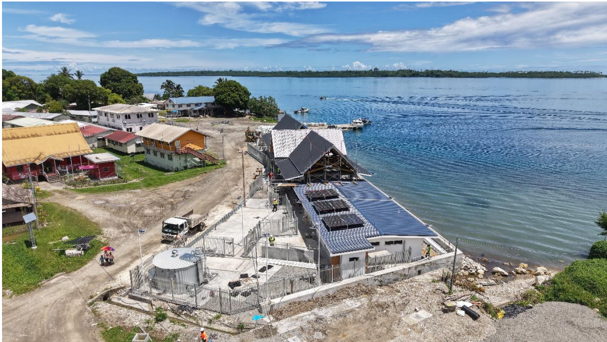
Photo 1 – The solar and battery system at Buala Market will support clean, renewable power to essential services event during extended periods of rain.
