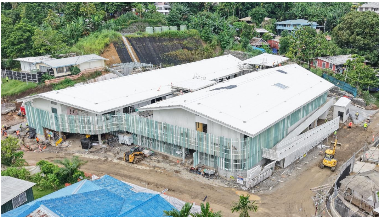
Photo 2 – Building shading and cross-ventilation will keep Naha Birthing and Urban Health Centre cool, while 350 solar panels installed on the roof will power its daytime energy needs.
